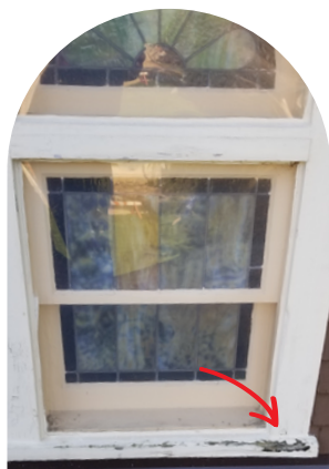
Small exterior windows on the northwest side of the building in need of repair.
