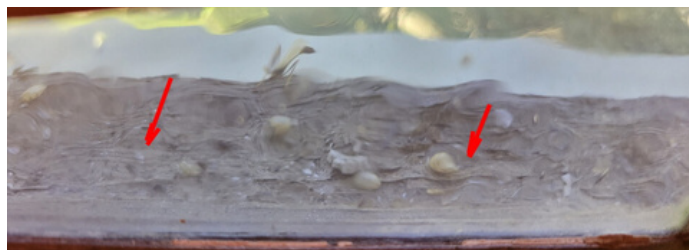
Webster Street windowsills (visible from the inside) shows peeling, cracking, and rotting wood.
