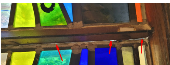
Light coming through gaps show that our three large stained glass windows facing Webster Street are sinking into the sill.
