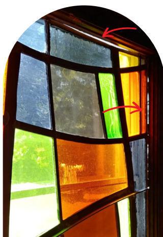
Window on southeast side of sanctuary is coming out of its frame.
